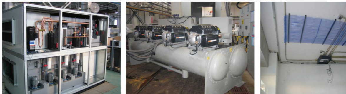
Temperature and humidity independent control air conditioning
