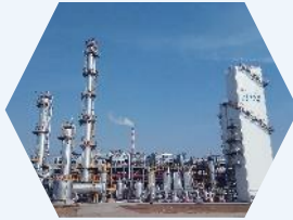
▲ Liquefaction plant/wellhead skid-mounted equipment ▲ Onshore wellhead gas treatment and processing
