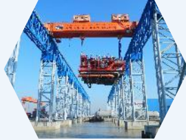
▲ Offshore oil and gas processing module
