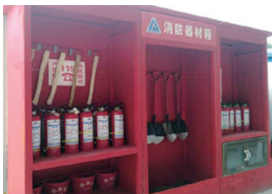
Figure 6: Firefighting equipment at a construction site
