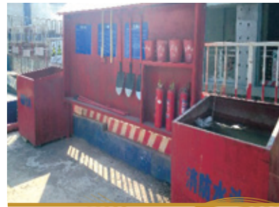
Fire fighting facilities
