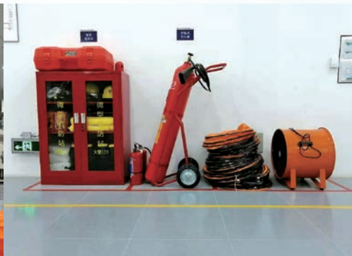
Micro fire station
