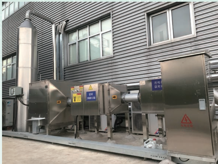
Organic waste gas treatment system
