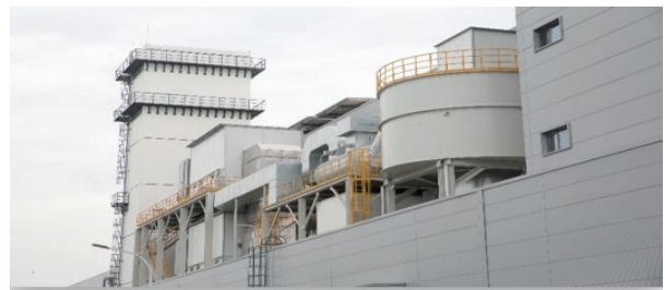
Exhaust gas treatment system
