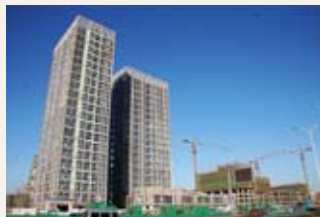
Tianjin Hailrun Plaza
