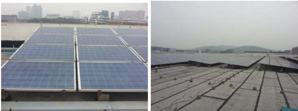
Figure 6.4 Photovoltaic (PV) Module Arrays
