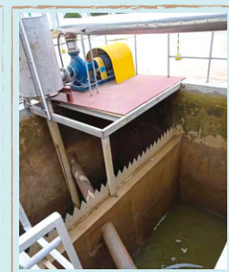
Water backwashing tank
