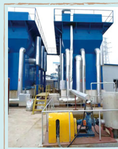
Original purification equipment
