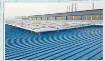
Solar heating plates
