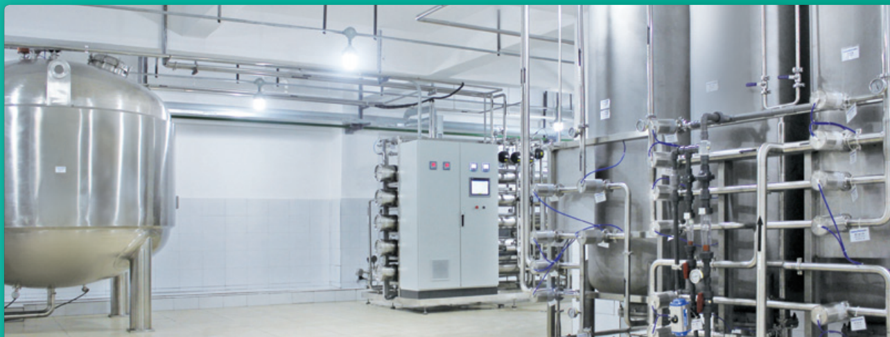
重慶康樂製藥有限公司（「重慶康樂」）— 廠區純化水系統 Chongqing Kangle Pharmaceutical Co., Ltd.* (“Chongqing Kangle”) — Water purifying system in the plant
