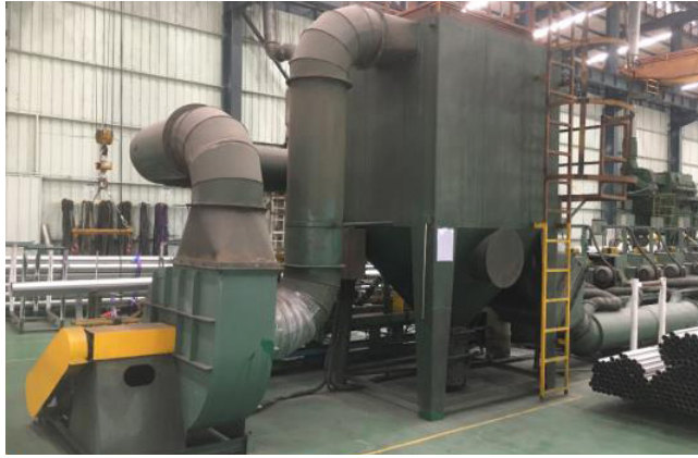
Production plants equipped with dust collectors with pulse jet filter bags
