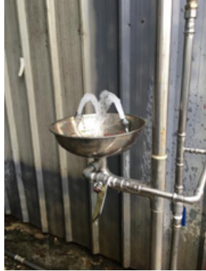
Figure 1: Fixed emergency shower head
