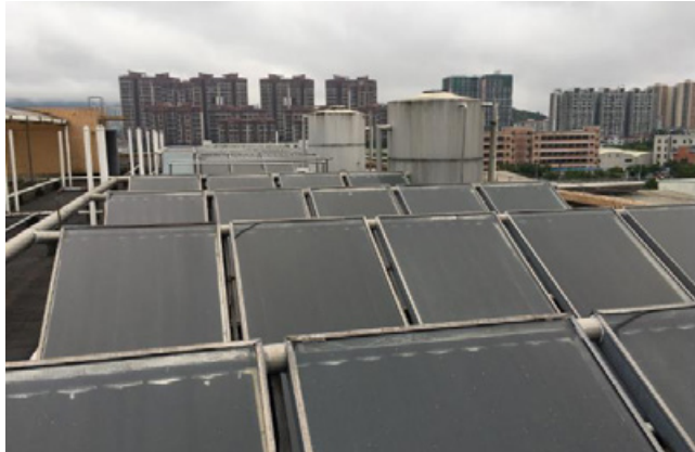
Solar energy equipment on the rooftop of staff quarters
