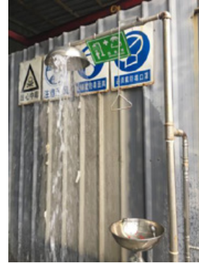
Figure 2: Fixed emergency shower head
