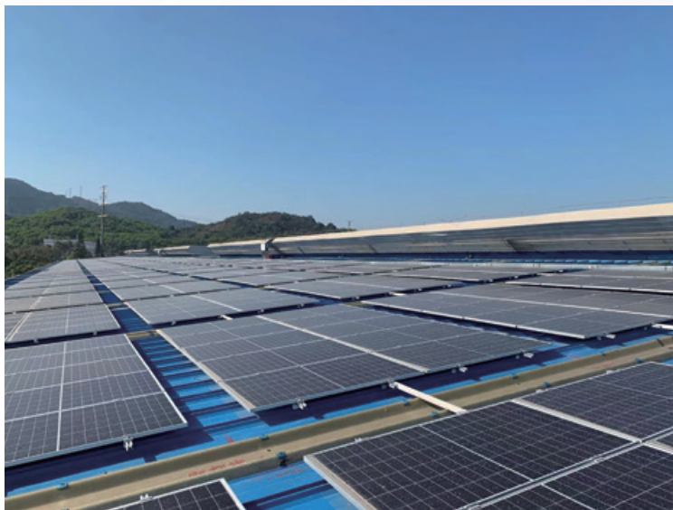
Solar panels on the rooftop of a production plant 生產廠房屋頂的光伏發電設備
