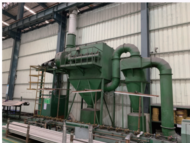
Production plants equipped with dust collectors with filter bags 生產廠房中設有布袋除塵器
