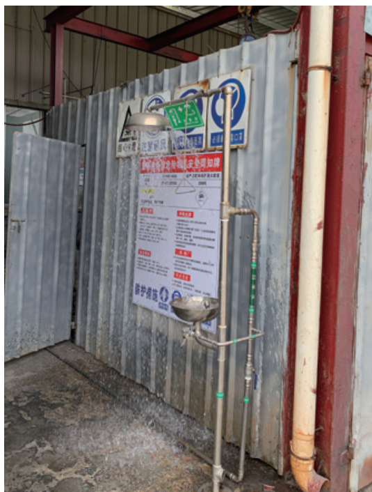
Fixed emergency shower facilities 固定式緊急沖淋裝置
