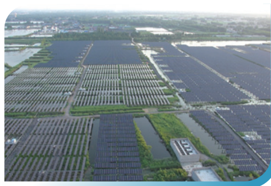
Centralised Photovoltaic Power Plant, Weishan County, Shandong Province
