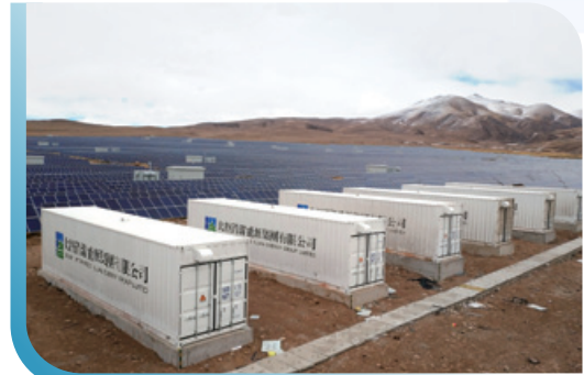
Photovoltaic energy storage project in Yangyi, the Tibet Autonomous Region
