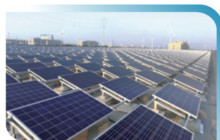
Distributed Photovoltaic Power Plant, Shandong Province
