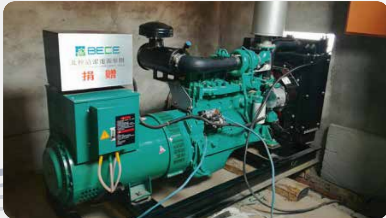
—The power generator donated to the Shanxi Datong Anjiazao School ——為山西大同安家皂學校捐贈的發電機
