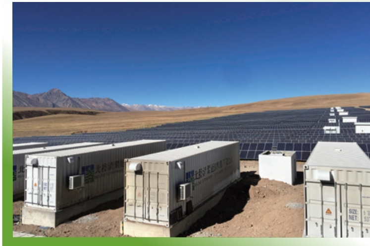
Yangyi Photovoltaic Energy Storage Project, the Tibet Autonomous Region 西藏自治區羊易光伏儲能項目
