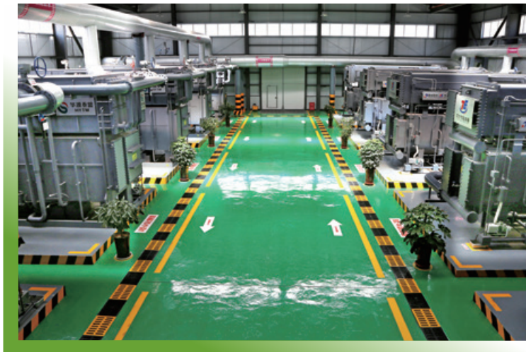
Clean coal consumption and power plant excess heat energy centralised heat supply project, Yinchuan City, the Ningxia Hui Autonomous Region 寧夏回族自治區銀川市清潔化燃煤及發電站餘熱能源集中供暖項目
