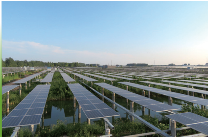
Centralised Photovoltaic Power Plant, Weishan County, Shandong Province 山東省微山縣集中式光伏發電站
