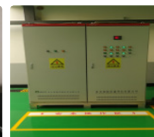
Positioning for power distribution
