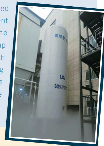
Ultra-low Emission Equipment of Coal-fired Boilers
