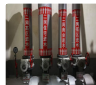
Signs for piping valve
