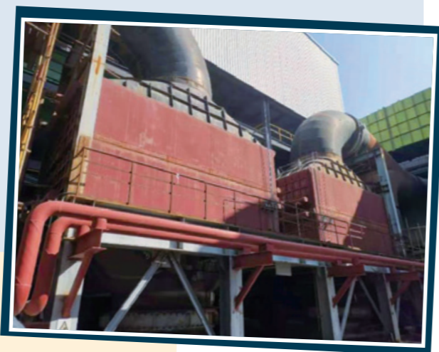
Heat Supply Recovery Device
