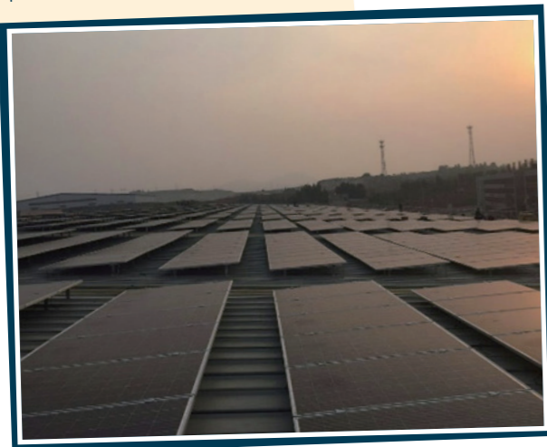
Mengcheng rooftop distributed photovoltaic power plant
