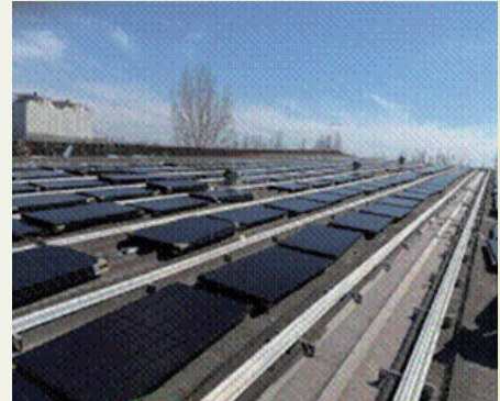
Photovoltaic power systems of the integrated smart energy project for COFCO Grains & Cereals
