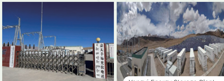
Yangyi Energy Storage Plant
