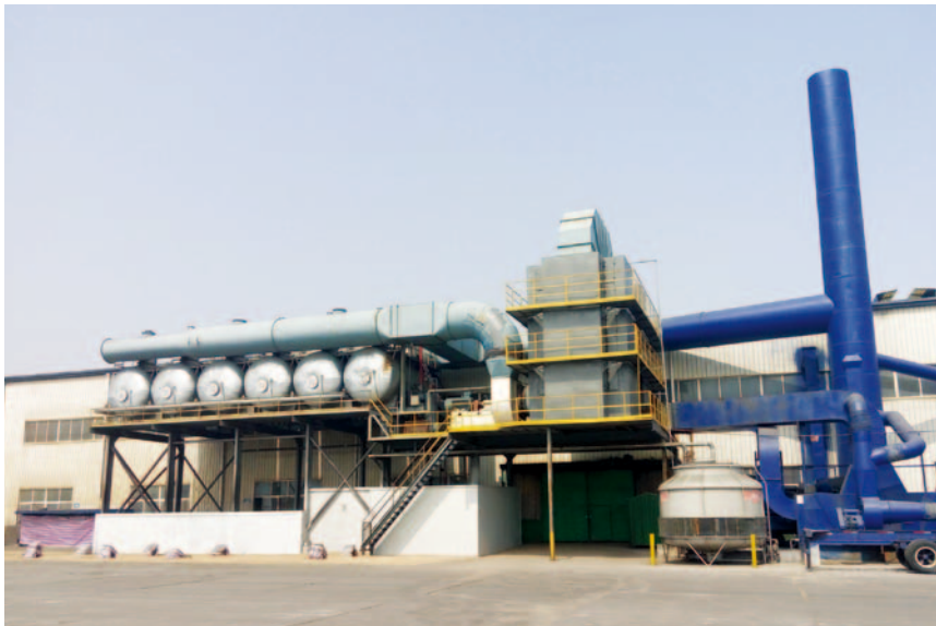
The organic solvent recycling system in Qingdao plant
