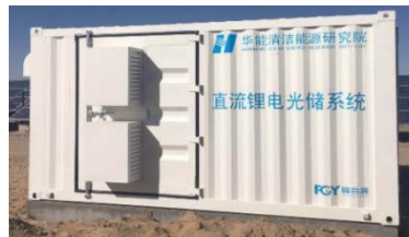
Energy Storage Containers
