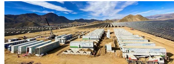
Renewable energy inside containers
