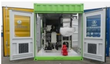
Power Generator Containers
