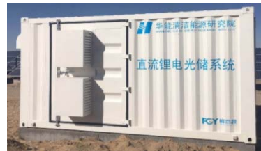
Energy Storage Containers
