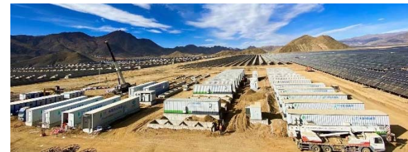
Renewable energy inside containers
