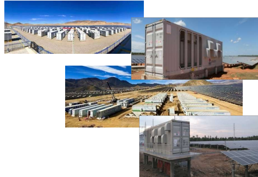
renewable energy inside containers
