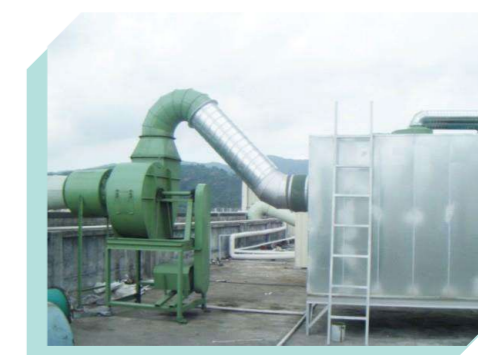
Newly built VOCs treatment facility
