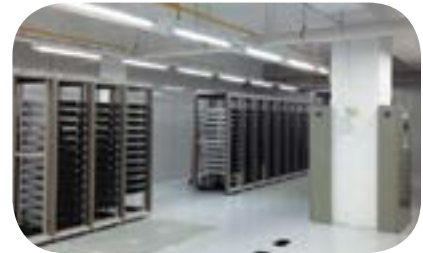
Anyang HTA High Temperature Data Center Interior
